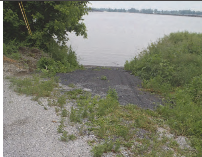
Photo 1. Some visible evidence of gravel from road washing down boat launch into lake.
