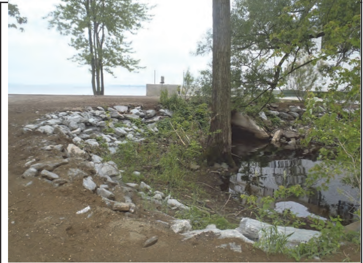
Photo 2. Evidence of sediment leaving site and being washed into Lake Champlain.
