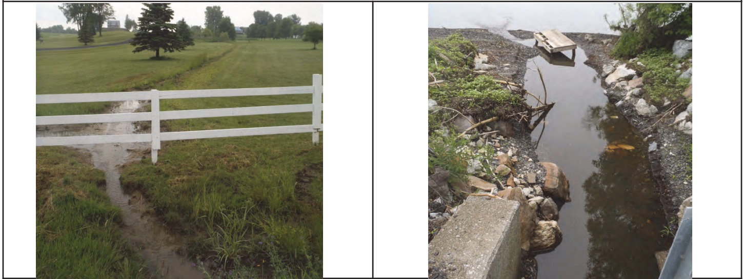
Photo 1. Active erosion above culvert.
